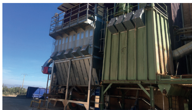
Figura 13. Interior de silos, tolvas, etc.
